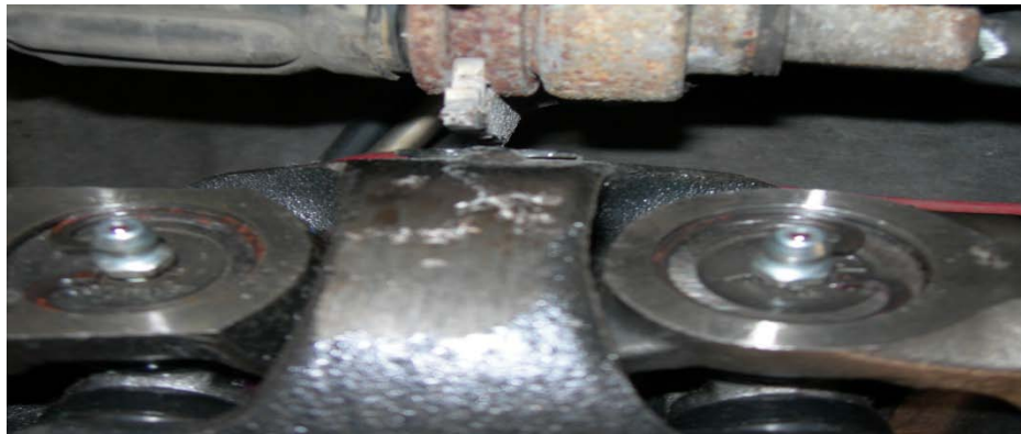
Figure 5. Different camera angle on the cleared shift cable bracket.
